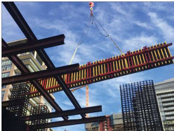
The forms are crane handled for the initial pour, but become part of the Self-Riser System for the remaining stories.
