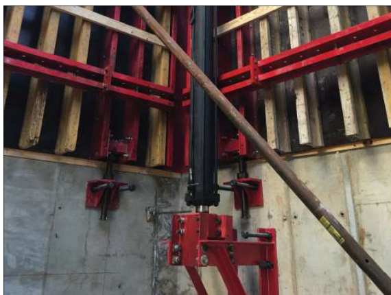
Hydraulic cylinders attach to a landing bracket anchored to the interior wall of the core.
