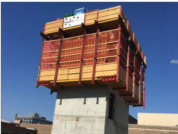
With the flip of a few switches, all interior and exterior formwork rises to the next level.
