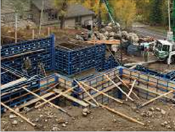
More dado slots along the side rail provide alternate tie locations “stepping” forms.
